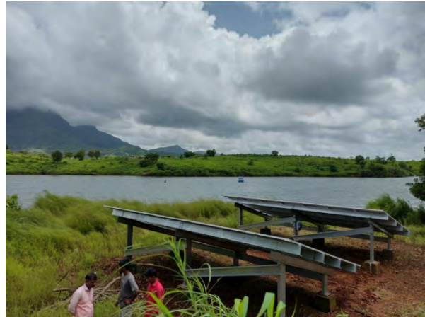
Image 3: Solar panels for line 5, Poshera
