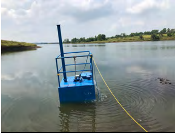
Image 2: Floaters attached to the water pump
